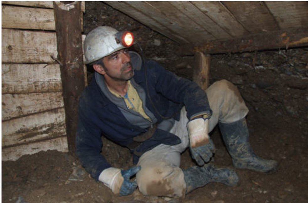
Photo 4 The supported overhead and walls of the chamber of the hallway, above the excavated T-2 megalith in the Ravne tunnel – with leader of the mining team, Enver Hasic, M.S. (photo by Islam Cero, June 17, 2006)
